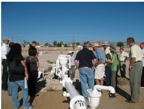
West Central Well Field
